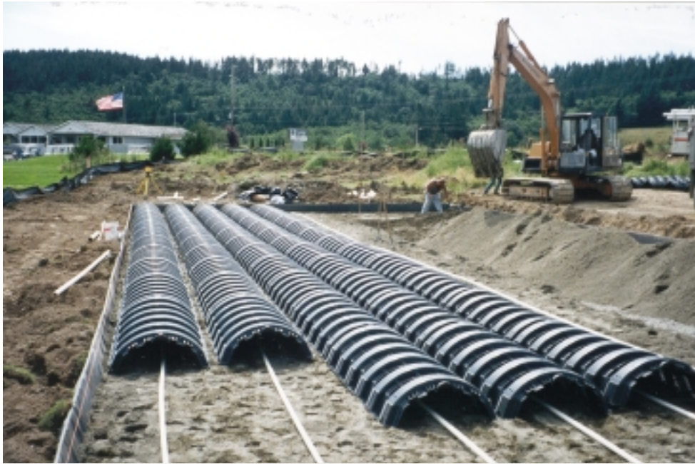
The standard septic system provides effective treatment, requires minimal maintenance, offers longevity and is a good economical choice for onsite wastewater treatment.
